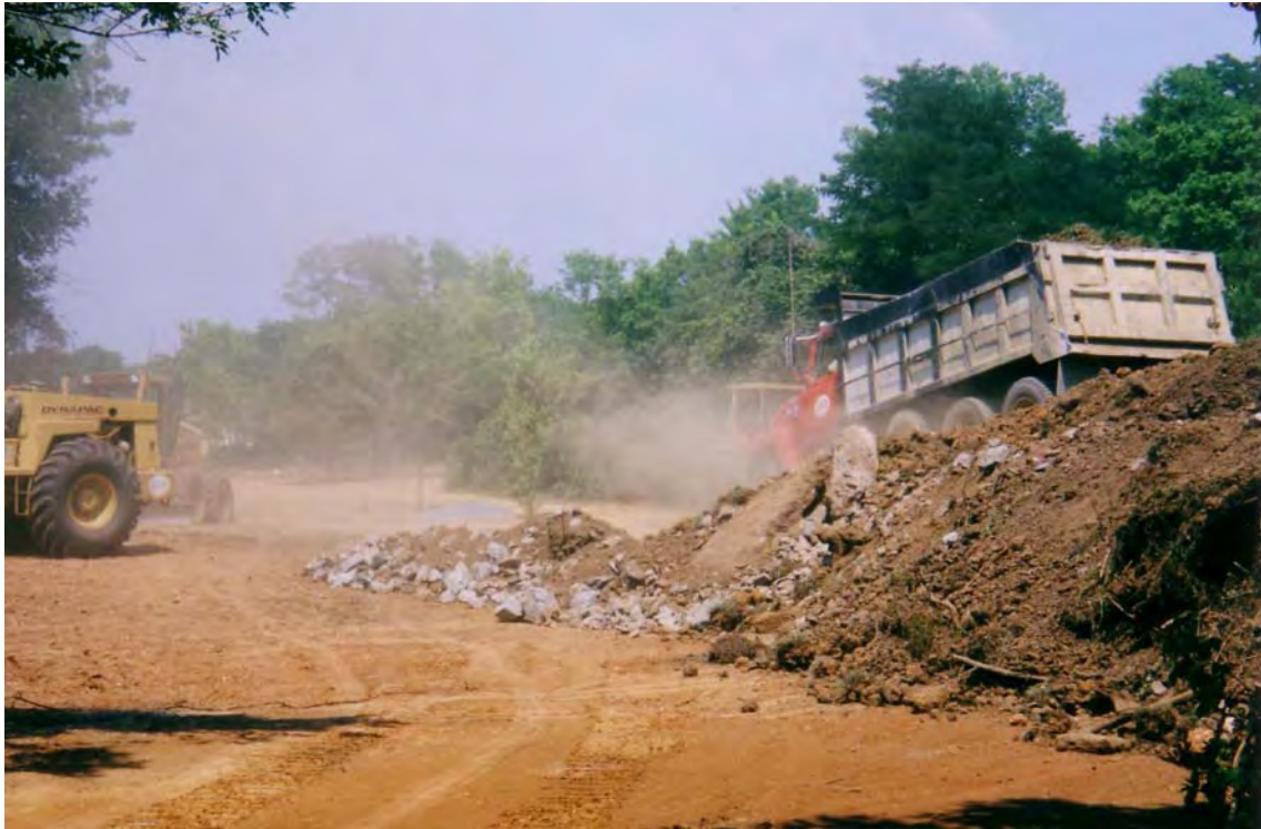
FIGURE 16. Photos of greenway construction in another part of Chattanooga. Notice the changes in surface soil conditions that must be considered if a greenway is to be built in an area with soil contamination. (photo: David M. Borowski, TDH, 02/13/06)
