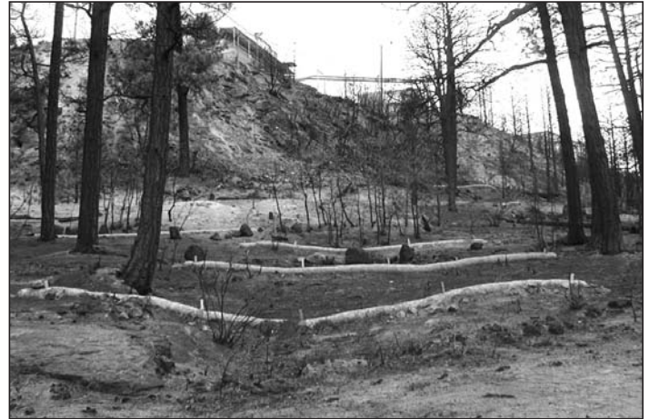
These straw wattles at Technical Area 46 are an example of "best management practices" action to control runoff in the aftermath of the Cerro Grande Fire. Photo by Steve Veenis, Water Quality and Hydrology (ESH-18)
