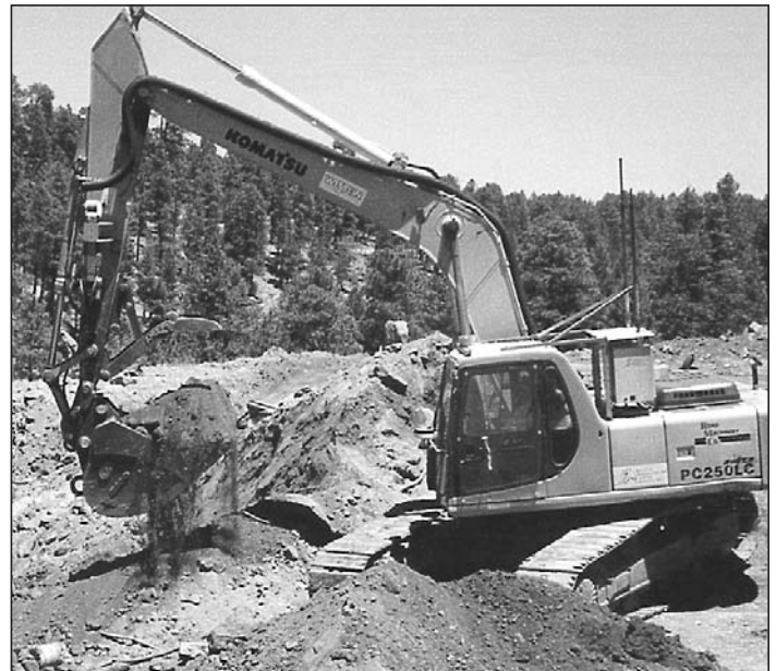
A remote excavator at work at Material Disposal Area P. An operator 200 feet away in a blast-protected building controls it. Video cameras on the machine show the operator exactly what he is digging into. Photos courtesy of Environmental Restoration Project Office (E-ER)
