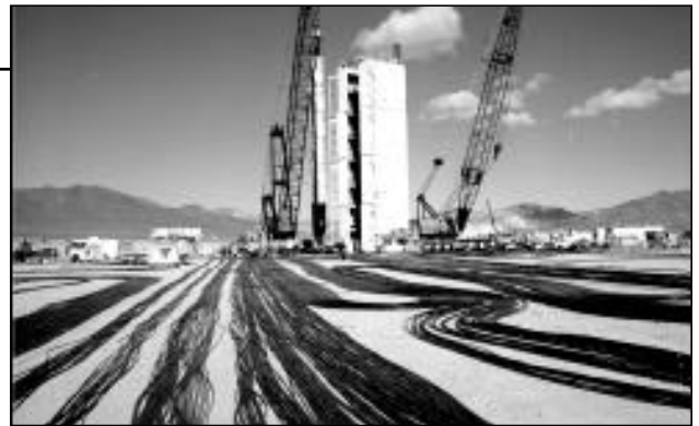
Signal cables spread across Yucca Flats, the principal underground nuclear weapons testing area at the Nevada Test Site. The tower, which was used to mount instruments in the canister suspended from the crane, will be removed before the detonation. The cables will be lowered downhole with the canister and then relay data to the surface. Photo courtesy of the U.S. Department of Energy
