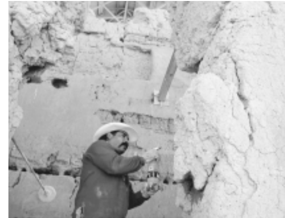
The National Park Service's Vanishing Treasures program seeks to address the preservation needs of archeological/architectural sites at national parks in the arid West. The program's targeted funding is helping to expedite restoration of sites like 700-year-old Casa Grande, shown being repaired by mason Ray Madril. (Photo courtesy of the National Park Service)
