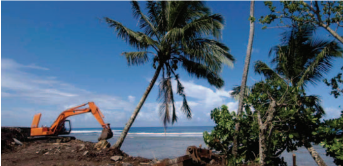
Excavator clears a section of land. Photo: Richard Murphy, Ocean Futures Society
