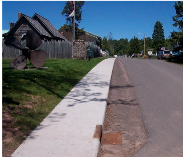
The La Pointe storm sewer project impacts mostly developed land and aims to improve runoff and drainage in areas including this street adjacent to the Madeline Island Historical Museum.
