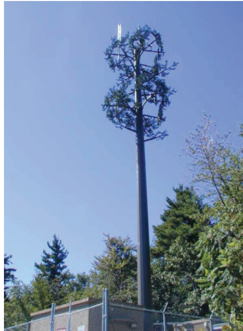
Disguised as a tree, the stealth monopole construction is intended to minimize adverse visual effects.
