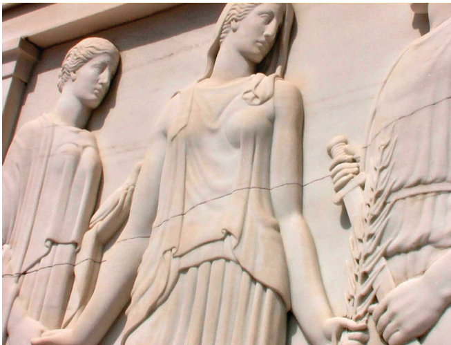
A view of one of the cracks in the façade of the Tomb of the Unknowns Monument
