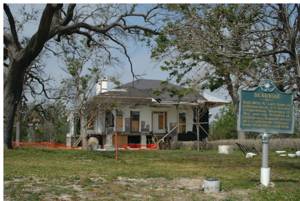
Beauvoir and the adjacent Jefferson Davis presidential library buildings are being repaired and rehabilitated in the wake of Hurricane Katrina. (courtesy FEMA)
