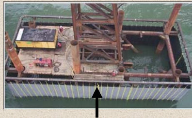
Acoustical Control Measure
