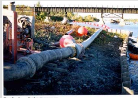
Photo No. 5: On-shore booster pump.
