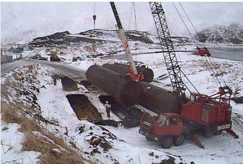
Figure 8: Temporary Tank Farm at Summer Bay Beach
