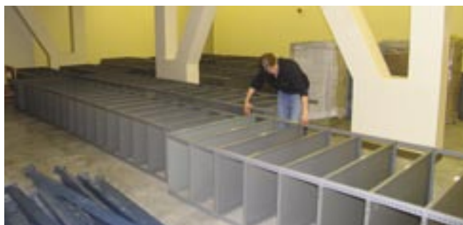
Shelving had to be purchased, assembled, installed, and cleaned before anything could go on it.
