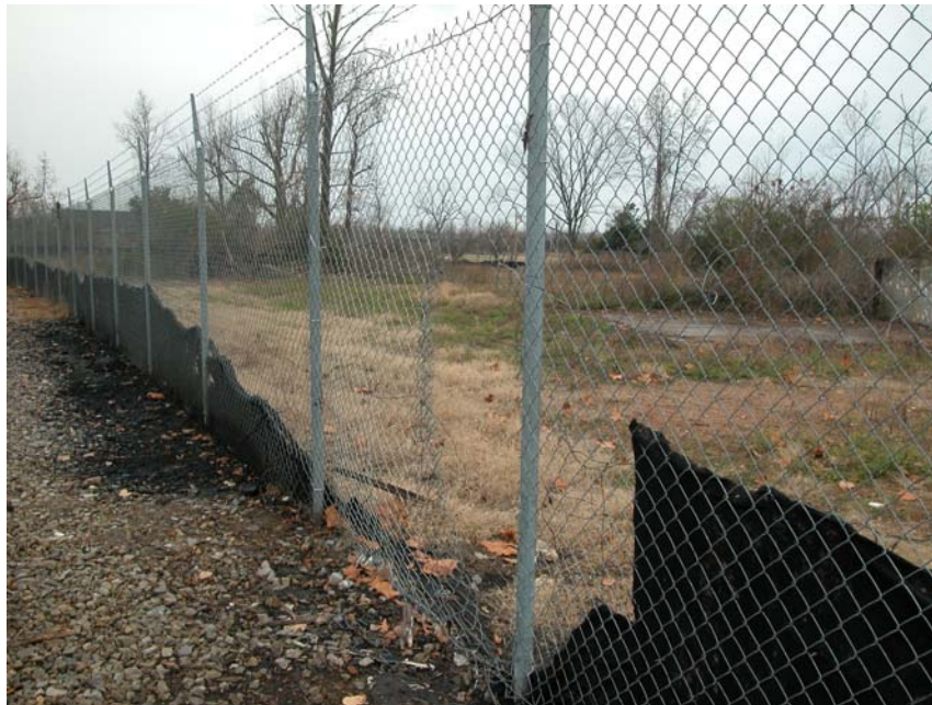
FIGURE 3. Photo of fence where it has been compromised to allow for trespassers to use the site as a shortcut (photo: David Borowski, 11/28/06).
