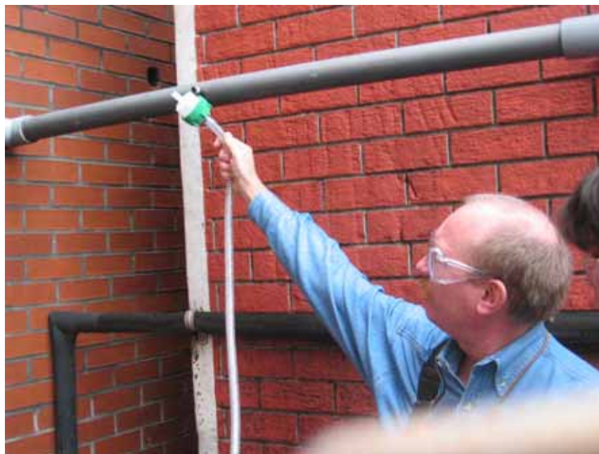
FIGURE 3 - EPA staff using the Lumex to analyze real-time air samples from the SVES exhaust pipe air-sampling valve. Duracell, Cleveland, Bradley County, Tennessee (Photo credit: Bob Safay, ATSDR, February 24, 2005)
