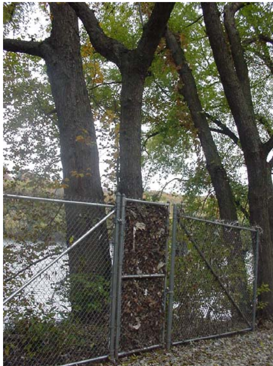
Photograph 12: Fence with flood debris on the western portion of the Crown Vantage Landfill site, August 11, 2005
