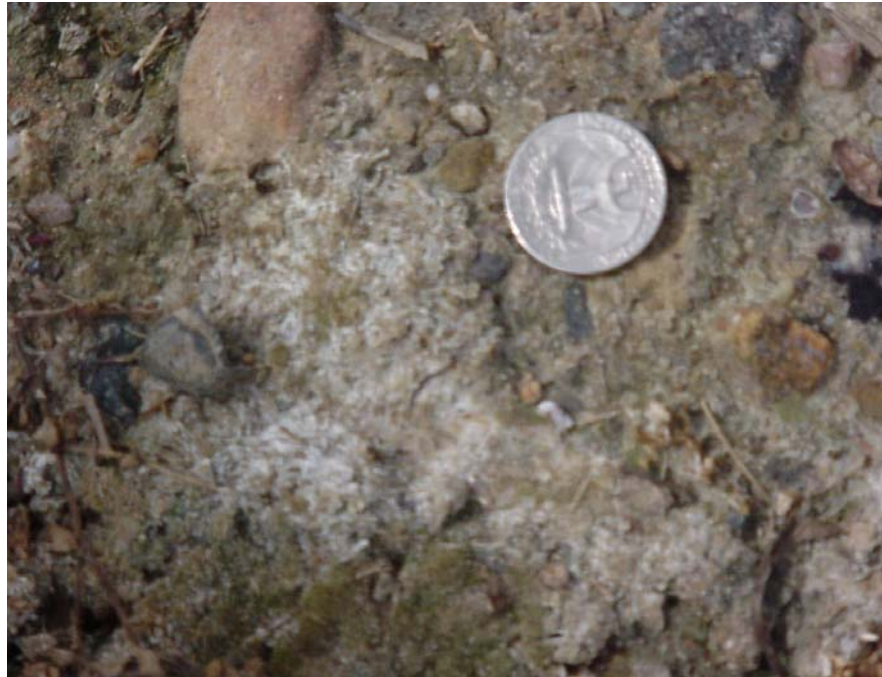
Photograph 3. Suspect asbestos contaminated soil
