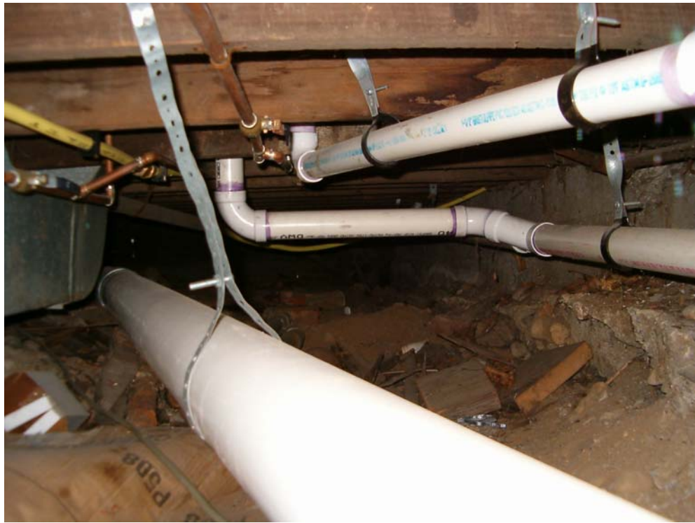
Basement crawl space area below former Rooms 2 & 3, former front office area and bathroom.
