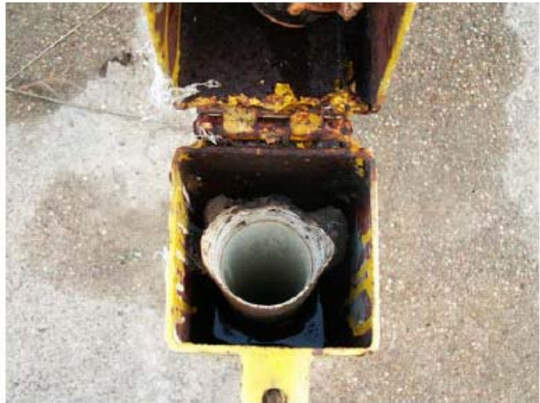
File Name: GSV_photo8.JPG Date/Time Taken: 01 Oct 2005 1733 Description: Warped top of riser pipe, well D-3R. N29°57'26.2"; W92°11'13.1"
