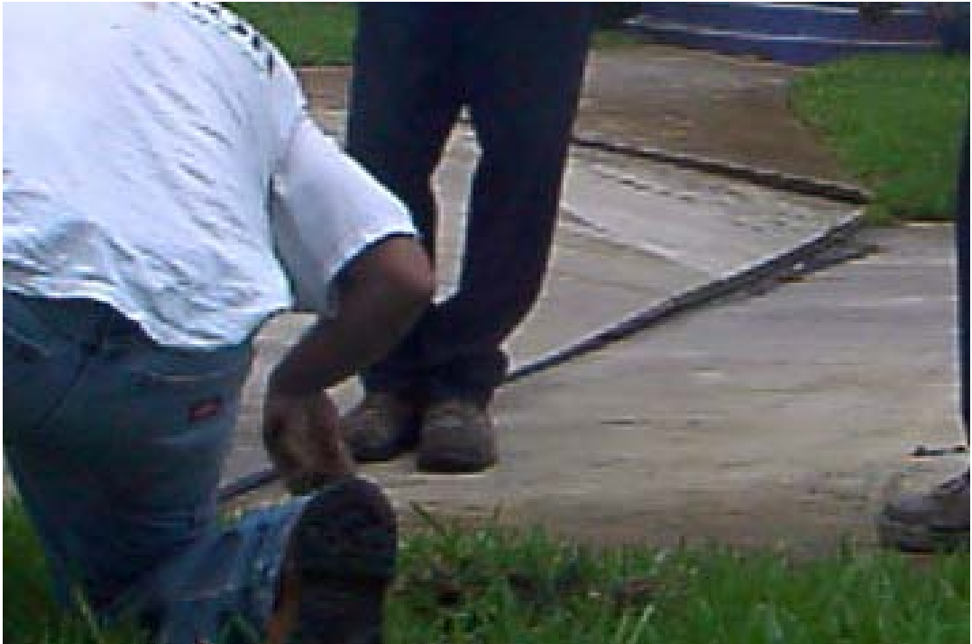
Photo 3: Structural damage due to subsidence in driveway.
