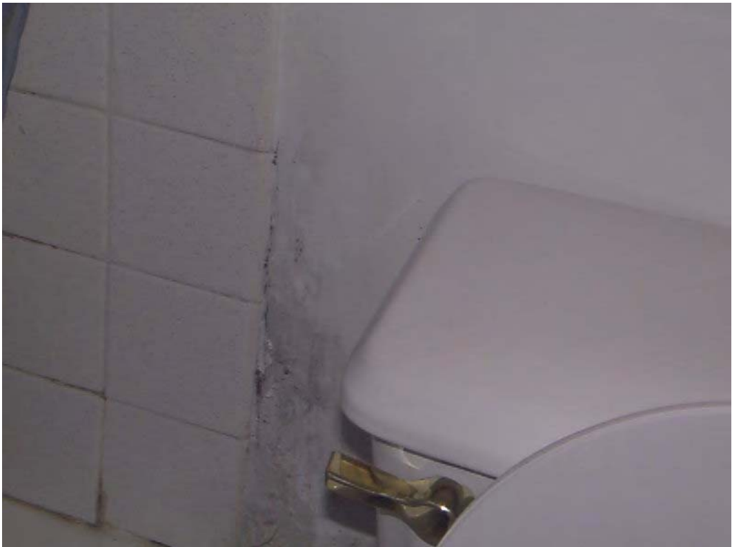
Photo 4: Attempted repair of wall crack inside Carver Square Subdivision home.
