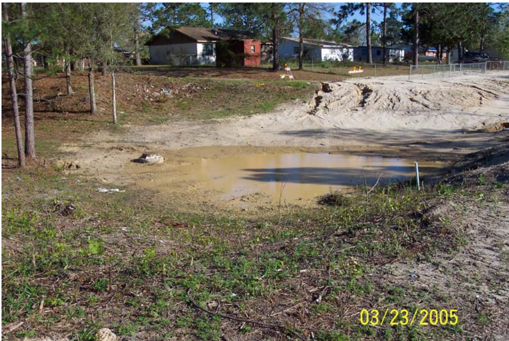
Photo 13: Collapsed sewer line south of Seventh Street. Residents report land subsidence and loss of parts of their yards.
