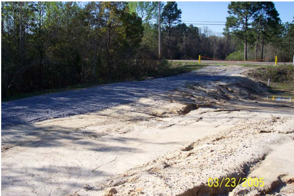
Photo 15: Closeup of land subsidence fill area looking north toward Seventh Street.
