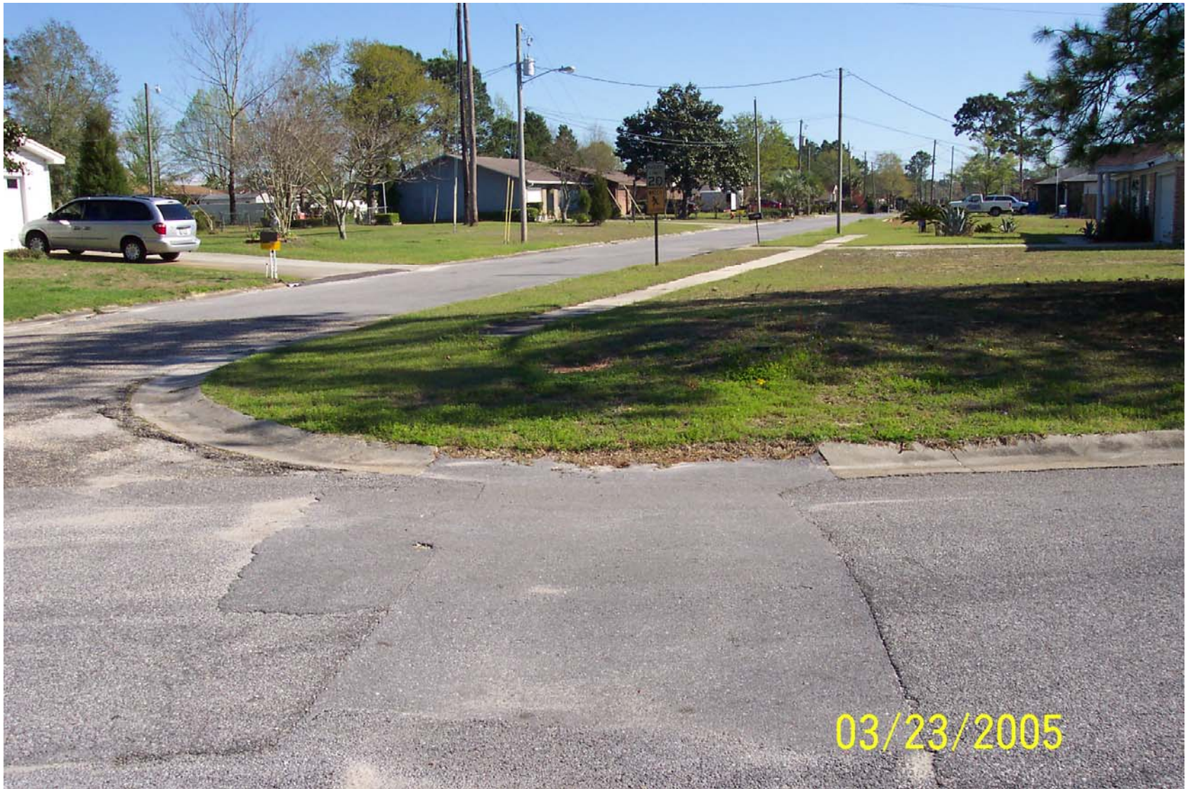
Photo 9: Corner of Flight Avenue and Joan Lane, pavement repaired for water main and gas line repairs. Residents reported a natural gas leak at this location in early 2005 required residents to evacuate their homes. Residents report the water main here (brown spot in grass) is repaired routinely for breaks.
