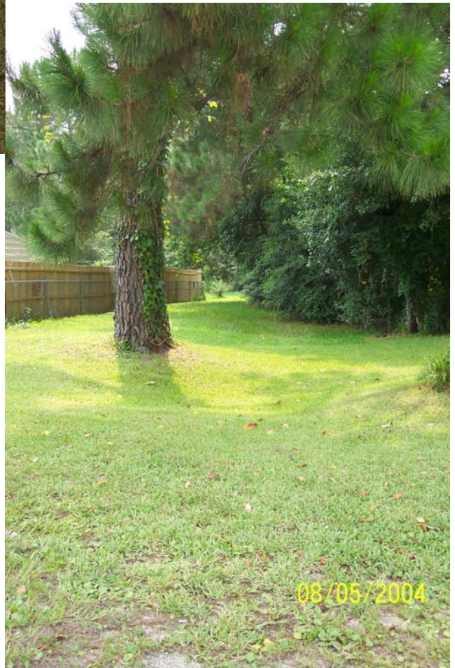
Photo 6: Another area of the subdivision with pronounced land subsidence.
