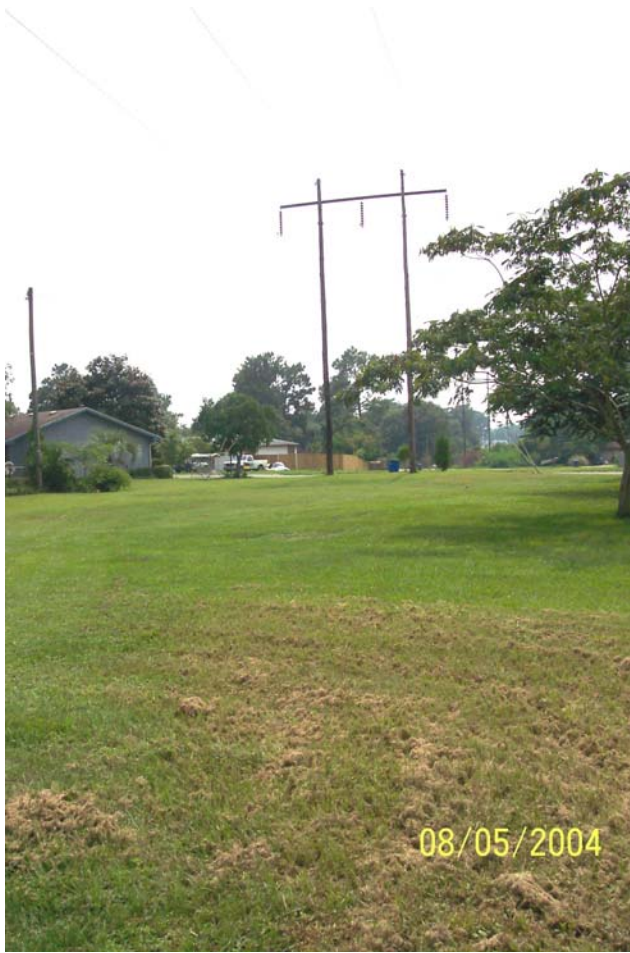
Photo 7: Another view of land subsidence in utilities easement.
