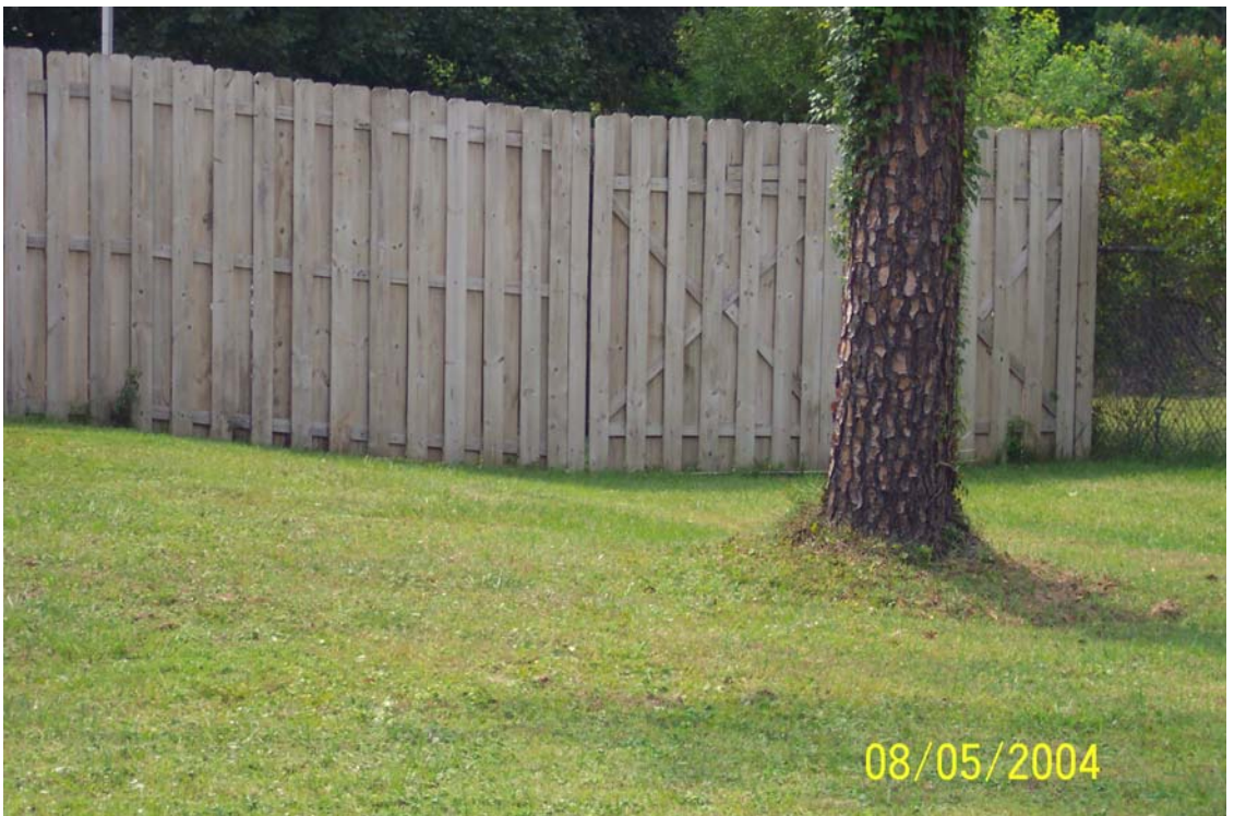
Photo 4: Flight Ave. area with land subsidence.
