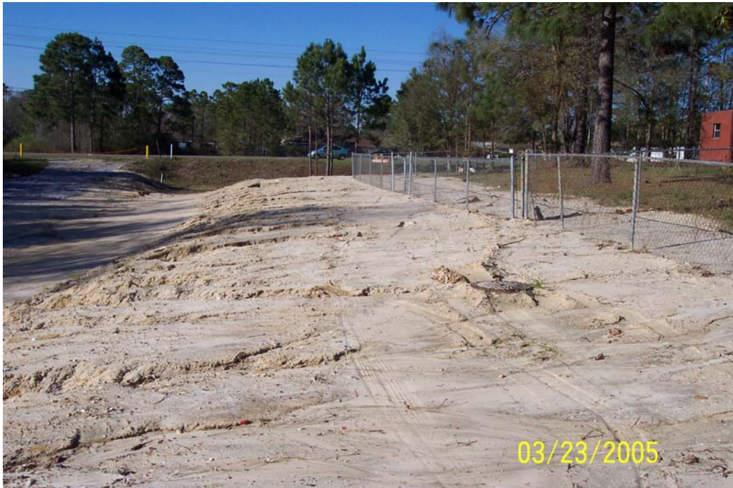
Photo 14: Land subsidence fill area looking north toward Seventh Street.
