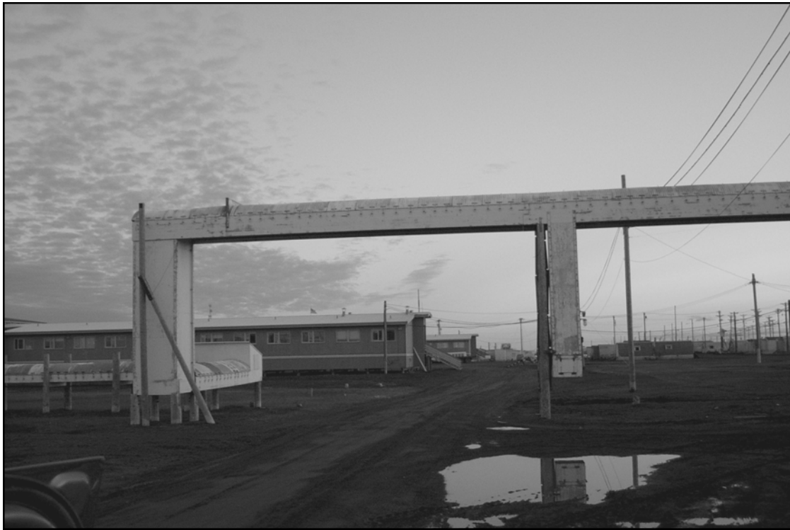
Figure 9. Utilidor in Barrow, Alaska.
