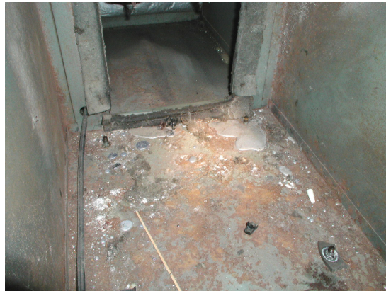
Mercury release in a home furnace on Princeton Avenue in Flint.
