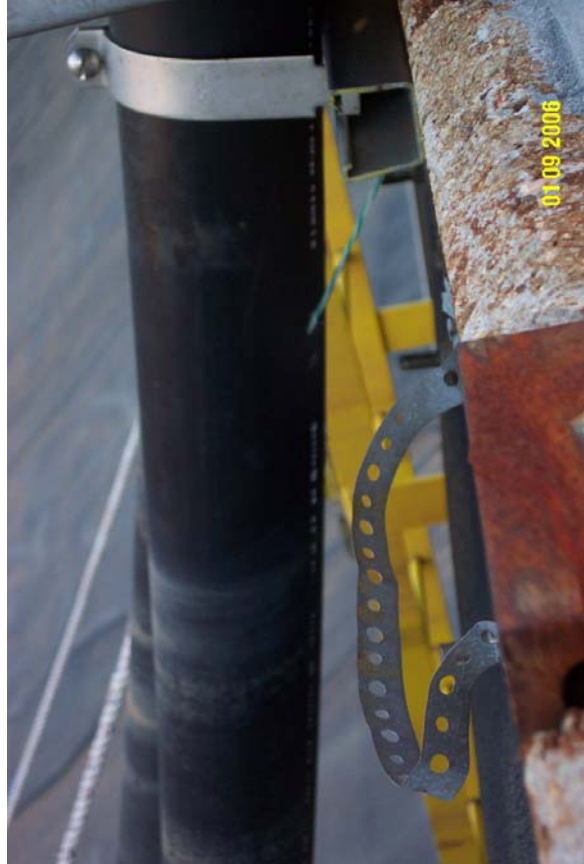
Figure 5.6 - High Water marks on HDPE Tubes
