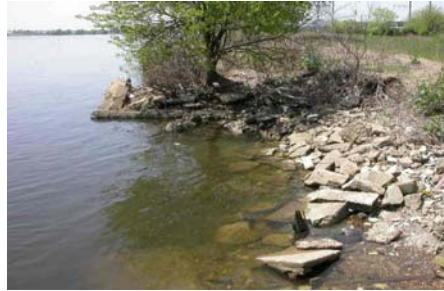
Unstable Shoreline at Lardners Point
