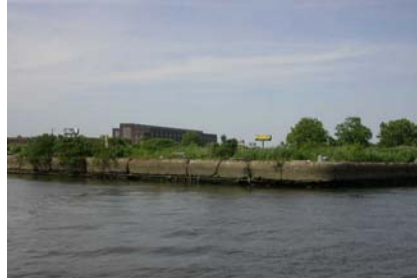
Failing Bulkheads at Old Phila. Piers
