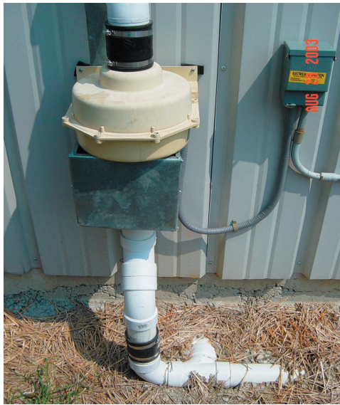
Installed mitigation system for PCE vapor at a business in Evansville.
