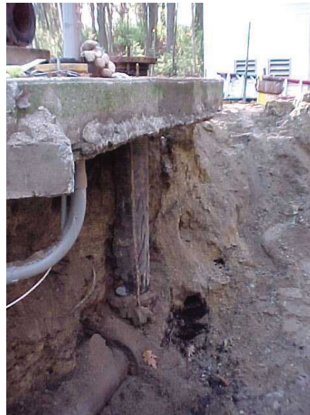
Pipe break undermined pump house — Nashua NFH, NH. USFWS Photo.
