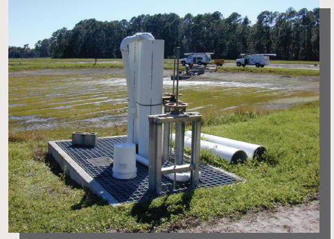
Water distribution structure — Welaka NFH, FL. USFWS photo.
