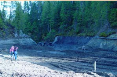
Removal of Cedar Creek Dam and channel restoration, restoring 12 miles of endangered bull trout habitat (Partners project in northeast Washington, Pend Oreille County)
