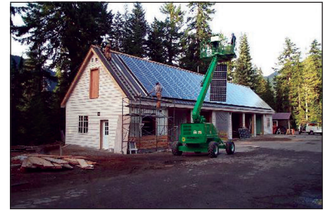
White River maintenance building at Mount Rainier National Park. Three hundred seventy-four photovoltaic panels provide 47 kW of power and reduce air pollution inside the park.
