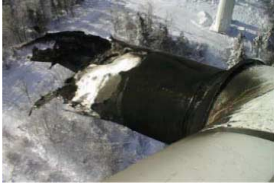
Figure 4. GMP/Searsburg Z40FS blade strike damage
