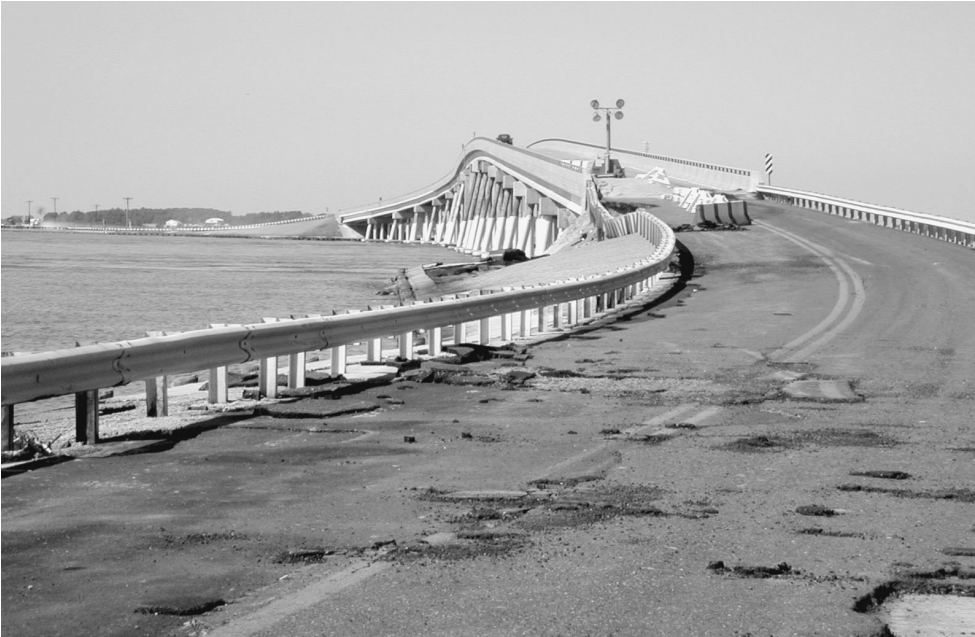
The damaging impact of Hurricane Isabel on Maryland roads and bridges has been significant. FEMA photo by Butch Ducote
