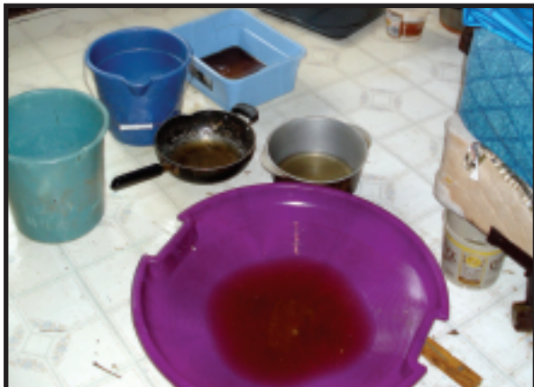
Containers collect water from ceiling leaks
