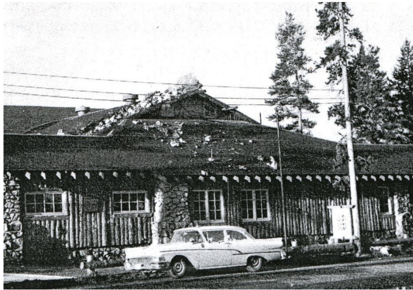
FIGURE 10: This is a photograph a collapsed chimney of the Union Pacific Dining Lodge in West Yellowstone, Montana. Chimneys collapsed on many buildings in Yellowstone National Park. A collapsed chimney at Old Faithful Lodge crashed through the roof and entered the dining hall. Had the quake come 4 hours sooner the hall would have been filled with the evening dinner crowd. (Witkind, 1964)
