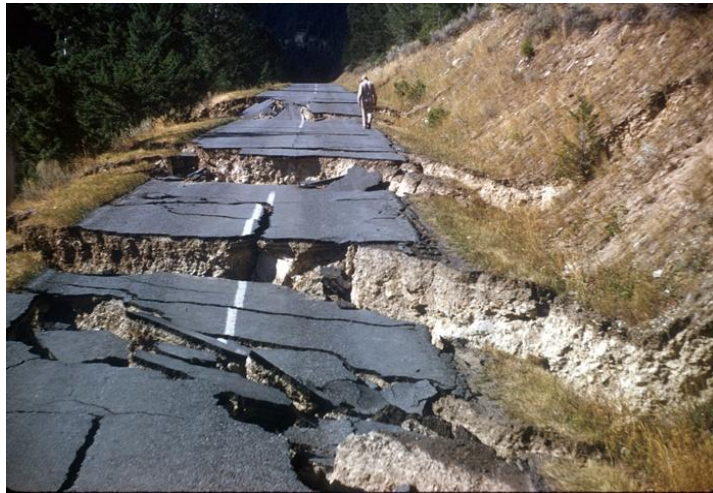
FIGURE 1: Photograph of fractured Highway 287: man inspecting damage. Hebgen Lake, Montana, Earthquake August 1959. (Colton, 2006)
