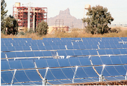
Arizona Public Service Company's Saguaro Generating Station is an example of solar trough technology. (Photo by Carol Shipman, APS)
