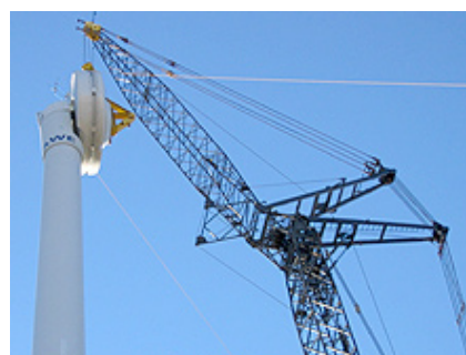
Construction crews hoist the hub into place on the Wray School District wind turbine. NativeEnergy's purchase of the unit's projected lifetime REC output made the project possible. (Photo by Wray School District)
