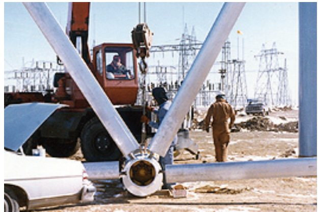
Gary Hoffmann worked on the Western crew that built a wind turbine in Archer, Wyo., in 1979. (Photo by Gary Hoffmann)
