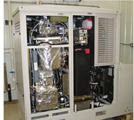
This PEM fuel cell installed at Haubenschild Farms is the first in the world to generate electricity from biogas captured from an anaerobic digester. (Photo courtesy of Philip Goodrich, PE)
