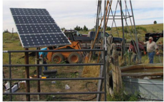
Engineering grad student Kala Meah (left) helps Robert Tarver and his father Bob Tarver (right) of Campbell, Wyo., install a 300-watt solar direct system. (Photo by University of Wyoming Electric Motor Training and Testing Center)
