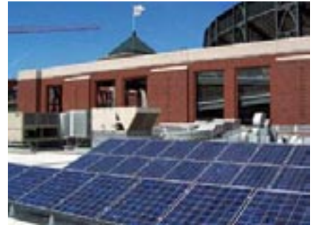
The 4.5-kW solar array Sharp installed for the San Francisco Giants Baseball Club helps power team offices and raises fans’ awareness about solar energy. (Photo by Sharp)
