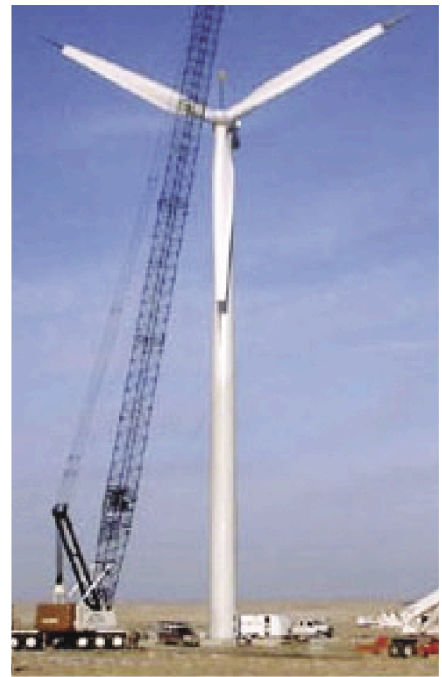
The 750-kW turbine on the Rosebud Sioux reservation is the first commercial wind turbine installed, owned and operated by an American Indian tribe. The turbine is connected to the grid at the Rosebud Casino and Hotel complex. (Photo courtesy of Intertribal Council on Utility Policy)
