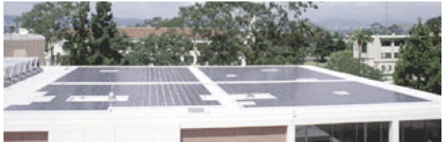
The solar array on top of LMU’s University Hall was the first of three rooftop systems PowerLight Corporation installed for the university. It generates between 230 and 240 kW. (Photo courtesy of PowerLight Corporation)
