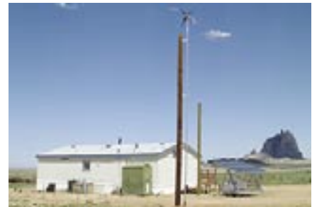
Navajo Tribal Utility Authority is using solar/wind hybrid systems to bring electricity to off-grid homes like this one in Shiprock, N.M. (Photo courtesy of NTUA)
