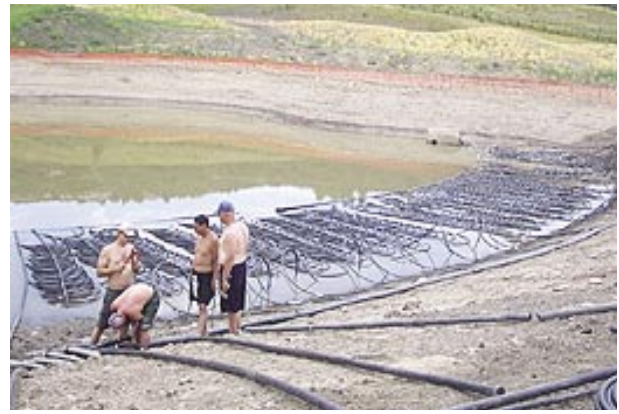
Technicians install the Ice Kube geothermal heat pump system for Snowmass Golf Clubhouse. ASC went to a Canadian company to find a unit that did not use ozone-depleting chemical in the condenser coil liquid. (Photo courtesy of Aspen Skiing Company)
