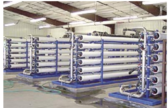
Four reverse osmosis pumps remove nitrogen and other impurities from Julesburg, Colo.'s well water. The purified water would leach minerals from the town's ductile iron water pipes, so it must be blended with well water to restore its pH balance. (Photo courtesy of Julesburg Utilities)
