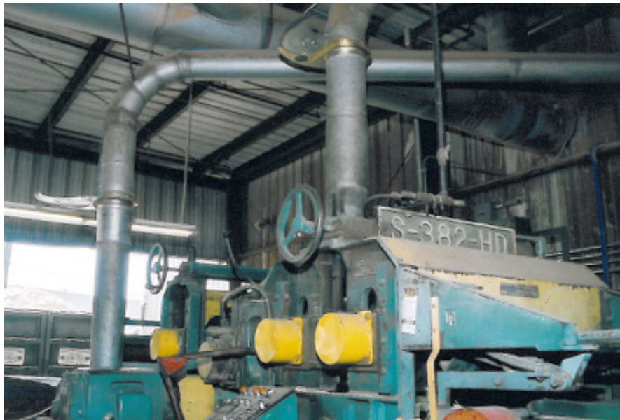
Heppner Hardwoods, Inc. took advantage of Azusa Light & Water's Business Energy Partnership Program to install a more efficient dust recovery system. (Photo by Steve Castro, Eagle Photography)
