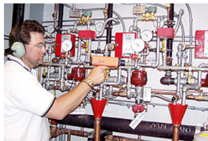
MRES Energy Services Technician Daryl Androli takes a reading on an HVAC system. MRES offers its members a variety of diagnostic services to help consumers gain control their energy use. (Photo by Missouri River Energy Services)
