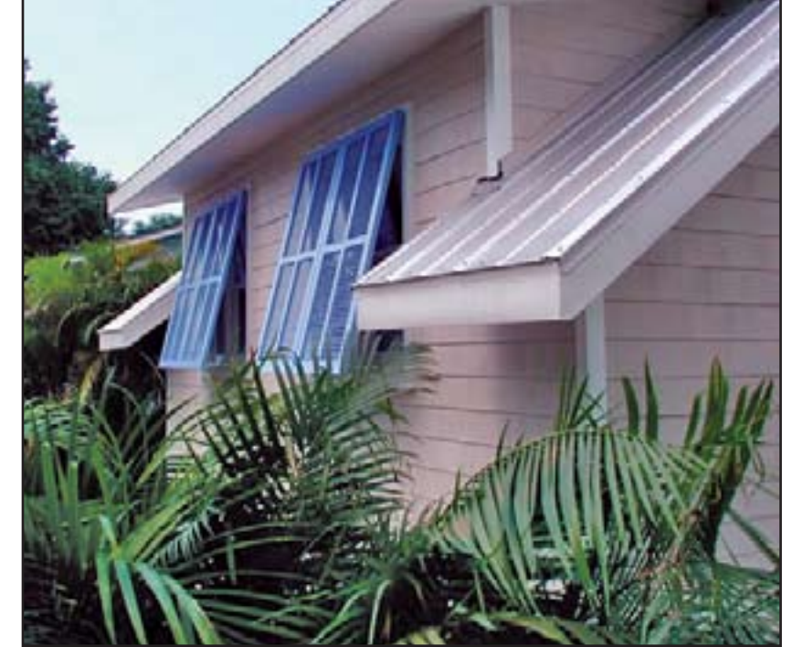
Homeowners were reimbursed for installing storm shutters, such as these pictured.
