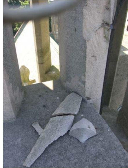
Figure 2.2: Stone spall at mechanical anchors
