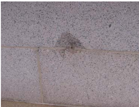
Figure 2.1: Mechanical anchor damage in facade
