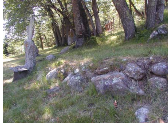
Double boulder wall before repairs
