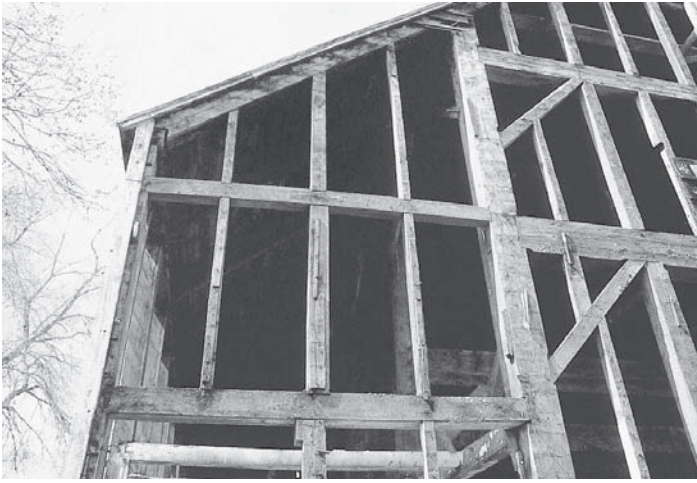
Sheathing direction determines the orientation of wall framing. This early-1800s barn (now dismantled) from Middleburg, N.Y., has studs to support wide clapboards. Note how braces take precedence over the studs.
