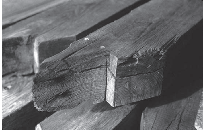
Rafters from a Great Barrington, Massachusetts, carriage shed showing a housed birdsmouth. This joint could be completely sawn.
