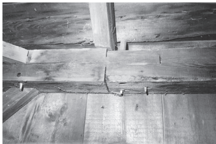
Simple bridled scarf in wall plate of five-bay barn 40 x 60 in Littleton, Massachusetts, built 1850-1870. The 2-in. tenon, 12 in. long, is secured by three pins. The builder used the same joint in the purlin plates.
