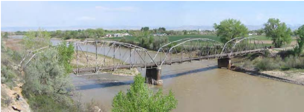
Figure 1.1. Fruita Bridge over the Colorado River, near Fruita Colorado. This three-span steel Parker truss was built in 1907. Each 47-meter (155-foot) span has eight bays. It has steel floor beams and timber stringers covered by a timber deck. Steel eyebars serve as bottom chords and principal diagonals and steel rods provide counterbracing. It served until a replacement bridge was built about one half mile downstream in 1970, and has been abandoned since then. The former wood railing has fallen away. The City of Fruita would like to reopen the bridge for pedestrian and bicycle use as part of a connecting bikeway leading to nearby tourist attractions, but has been stymied by the expense of rehabilitation. The north span, which was instrumented, is at the far right.
