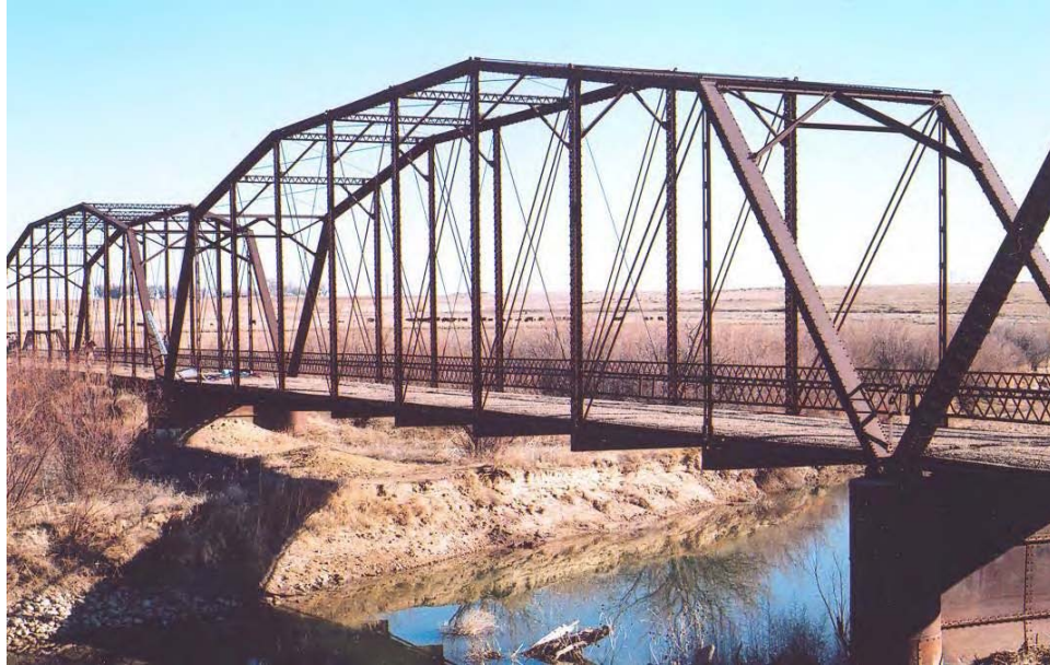
Figure 1.5. Prowers Bridge over the Arkansas River, near Lamar, Colorado. This bridge consists of one 5 panel Pratt pony truss built in 1921, three 9 panel Camelback Pratt through trusses built in 1909, two 6 panel Pratt through truss built in 1902 and 1906. The 49-meter (160-foot) Camelback Pratt through truss span, seen in this photo, was instrumented because it received the greatest wind exposure. It has steel floor beams with steel stringers, covered by a corrugated metal deck with asphalt pavement. It has steel eyebar bottom chords and diagonals with steel rod counterbracing. The railing is a steel lattice with single angle top and bottom rails. Virtually all paint has weathered away. It survived a major flood of the Arkansas River in 1921 and served as a highway bridge until its abandonment in 1994 when a nearby replacement bridge was constructed.
