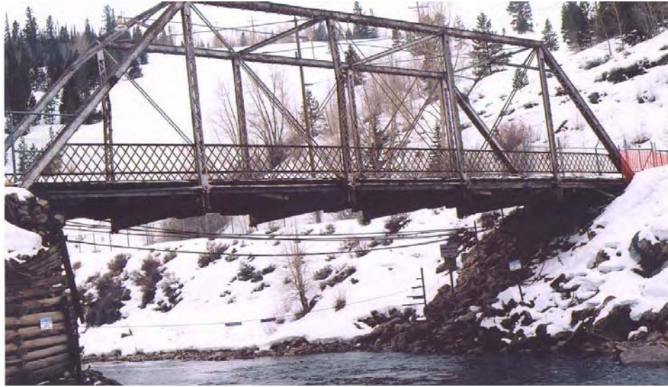
Figure 1.7. Blue River Bridge over the Blue River near Silverthorne/Dillon, Colorado. This 37-meter (120 feet)-span steel Pratt truss has five bays, with a timber deck on steel stringers. It has steel eyebar bottom chords and diagonals and steel rod X-bracing at the center bay. The railing is a steel lattice with double angle top and bottom rails. It is believed to have been built approximately 1895 as the Two-Mile Bridge near Breckenridge, Colorado and moved to this site at a later, but unknown, date. It is known to have been in its present location when the Dillon Dam was built immediately upstream in 1960. Closed to vehicular use, it is still used as a pedestrian crossing of the Blue River.
