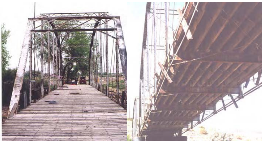
Figure 1.2. Fruita Bridge Deck. The deck timbers are spiked to timber stringers, which bear on steel floor beams. The deck is discontinuous in that there are gaps between the deck timbers. The short vertical timbers are the remnants of a former wood railing.
