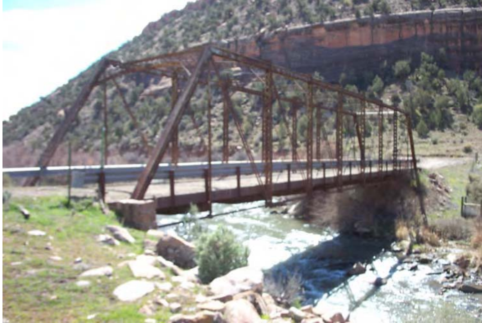
Figure 1.9. San Miguel Bridge over San Miguel River near Uravan, Colorado. This 43-meter (142-foot) wrought iron Pratt truss was built in 1886 as part of a five-span Fifth Street Bridge over the then Grand (now Colorado) River at Grand Junction, Colorado. One span was relocated to the San Miguel river location in the 1930's. It has a roadway of gravel on an unusual system of semi-circular lengths of corrugated metal pipe set between steel stringers. It has wrought iron eyebar bottom chords and diagonals and wrought iron rod counterbracing. A steel vehicular rail has replaced the original railing. It served the mining industry in western Colorado until the 1980's. Abandoned since 1990, it remains the oldest bridge originally built in Colorado.
