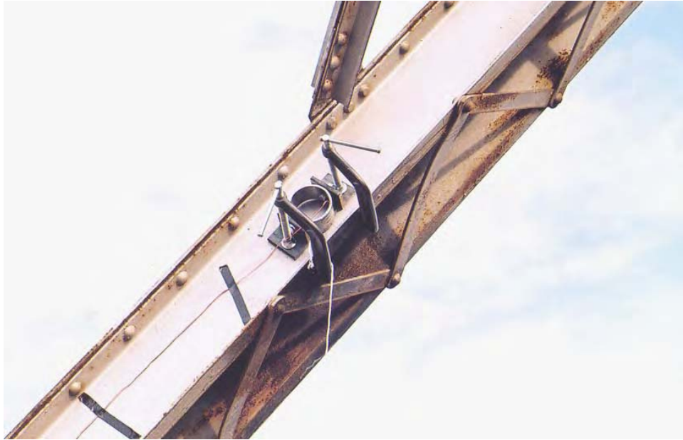
Figure A.9. Strain transducer installed on a portal at Fruita Bridge. It is located at the same elevation as the panel point of the portal's knee brace.
