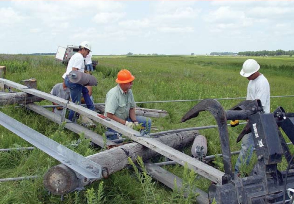
Left: Havre Line Crew Foreman Ron Barnett , standing left, joins Havre Lineman Ron Smith , and Glendive Lineman Ryan Staiger in wrecking out a wooden structure on the Pickert-to-Grand Forks 230-kV transmission line, which was damaged by tornadoes July 15, 2007.
