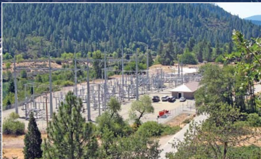
Left: An aerial view of Trinity Substation, September 2007.
