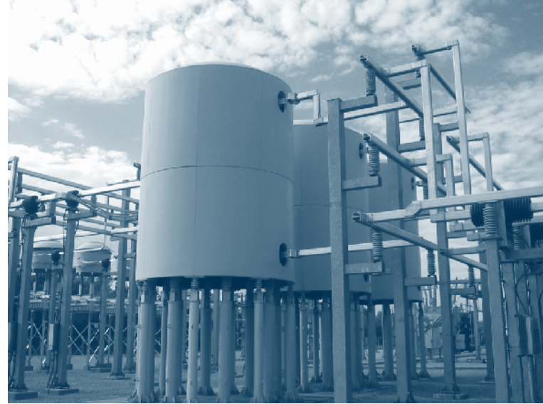
A static var compensation system, which Western has installed at the Watertown, S.D., Substation, was one of the technologies examined in the Dakotas Wind Transmission Study to determine how to mitigate overloads and stability problems when wind generation is added to the existing transmission system.
