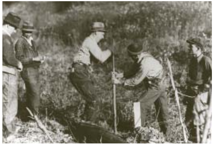
Early transmission line construction meant grabbing a shovel and digging a hole for each pole. (Photo courtesy of the Bureau of Reclamation)
