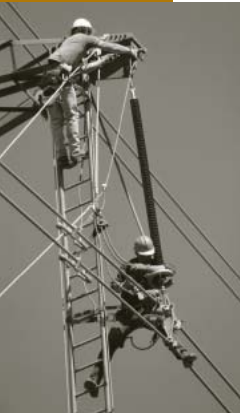
In 1993, three years after the Bears Ears-Bonanza line was completed, line crews from across Western worked together to replace insulators along the 101-mile line. Linemen like Sam Naill and Scott Westover worked from 6 a.m. until early evening six days a week to complete the massive job. (Photo by Dennis Schurman)
