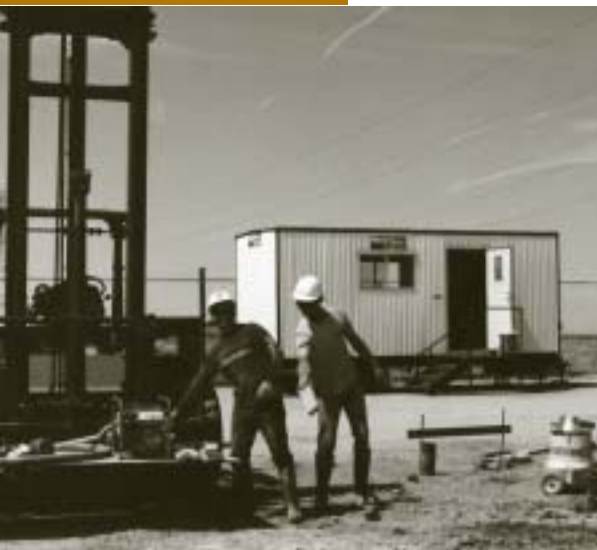
Crews begin work on the Maxwell Series Compensation Station as part of COTP.
