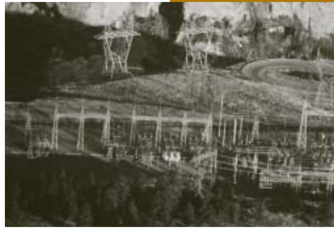
Reclamation retained ownership of the Yellowtail powerplant and switchyard after Western’s formation. (Photo courtesy of Harvey Hunkins)
