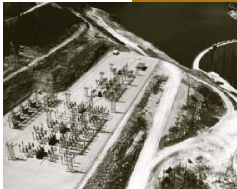
Switchyards connect the transmission grid with generating plants. (Photo by the Bureau of Reclamation)
