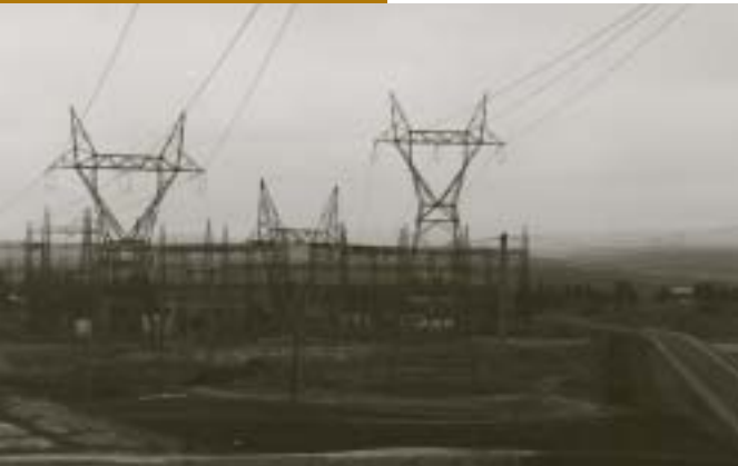
Tracy Substation was expanded to accommodate COTP transmission requirements.
