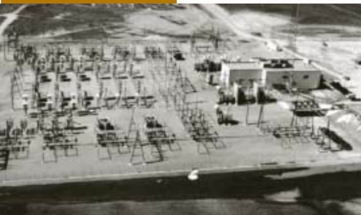
The Miles City Converter Station is used to transfer power between the eastern and western grids.
